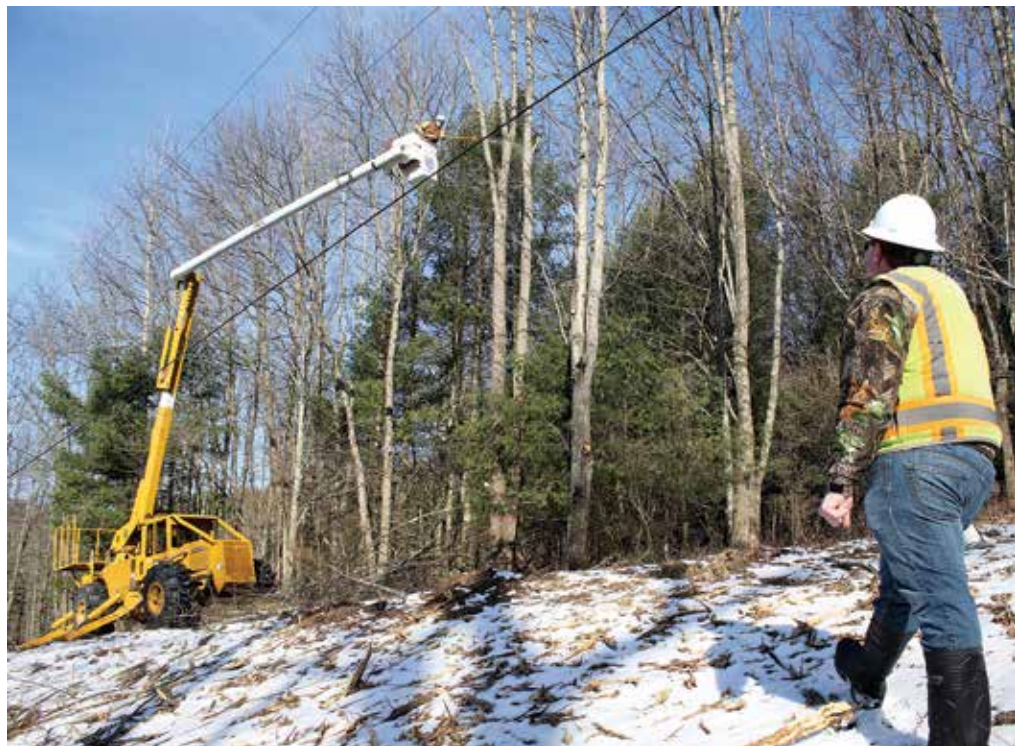
ASH PROBLEMS: Chris Cilino, a foreman with Asplundh Tree Experts, works to remove a dying ash tree on the Plank Road Substation circuit in Bradford County while forester Colby Marshall looks on. Because ash trees become very brittle as they die, the trees are taken down limb by limb, starting at the top of the tree, to ensure the safety of tree workers.
