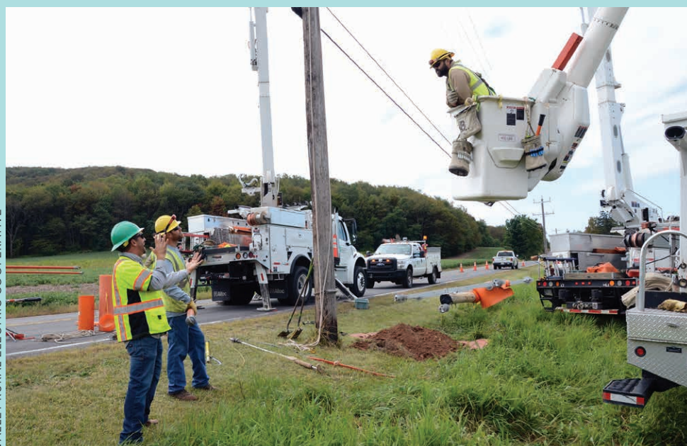
LEARNING WHILE WORKING: Fred Kuzemchak, left, a safety instructor with the Pennsylvania Rural Electric Association, provides on-the-job training at Huntingdon-based Valley Rural Electric Cooperative. He is shown with, from left, linemen Curt Wilson and Matt Fish.
