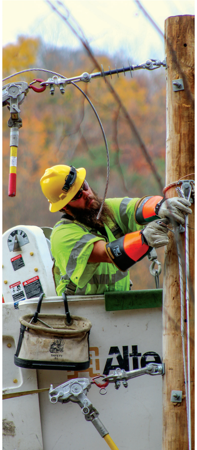
POLE PREP. Claverack lineman Jeremiah Lund readies a pole for new electric line during a line relocation project near Hop Bottom on Oct. 21, 2020. Linemen from all three co-op districts took part in the day-long project to relocate about 15 spans of line to improve access for crews as well as reliability for members.
