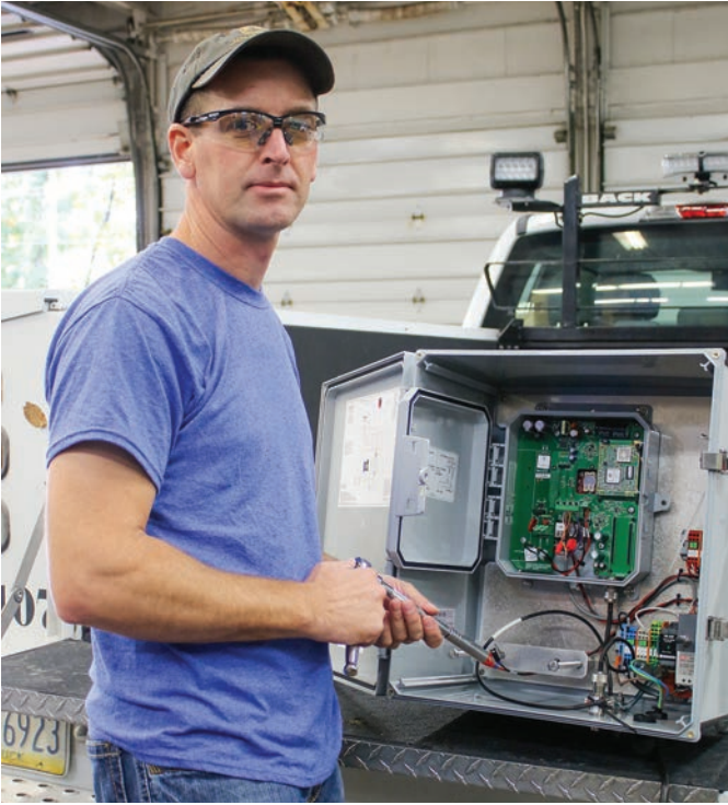
ADVANCED METERING. Claverack electronic technician Larry Beebe prepares networking equipment for installation as part of the co-op's advanced metering infrastructure (AMI) project that began in October 2020. The cooperative plans to replace all of the existing meters on its system over the next two years as part of the AMI project. The new wireless metering system will offer real-time meter-reading and outage-reporting capabilities.
