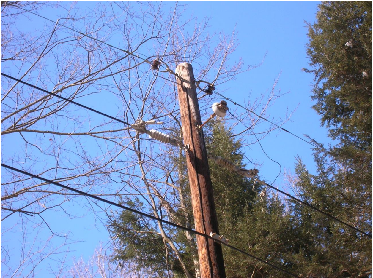
DOUBLE DEADEND, FEED THROUGH, TREE CABLE
